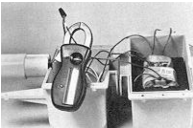
Short Circuit Lamp Current Test
